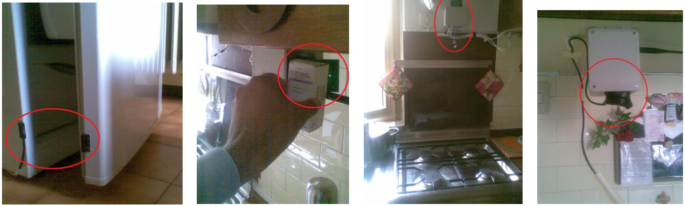
(a) Magnetic contact sensor on the fridge door (b) Passing a tagged medicine box over the RFID reader (c) A board with temperature sensor over the stove (d) Passive infrared presence sensor over the kitchen table
